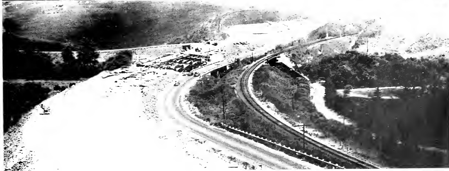
Views of reconstruction on Coast Highway west of Santa Barbara. Top and bottom scenes show Canada be Refugio bridge under construction. Here a plane re-alignment on a fill eliminates a long old and narrow old structure with restricted sight distance.
